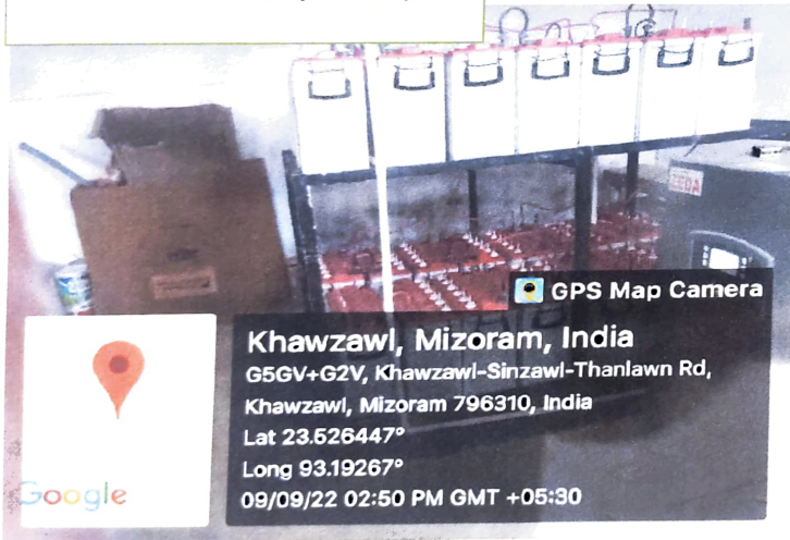
Solar Panel Backup Battery
